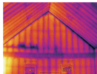
Insulation and Air Leakage
